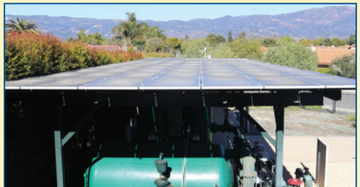
Solar panel roof at the District's San Ricardo Well
