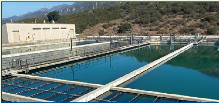
Corona Del Mar Water Treatment Plant
