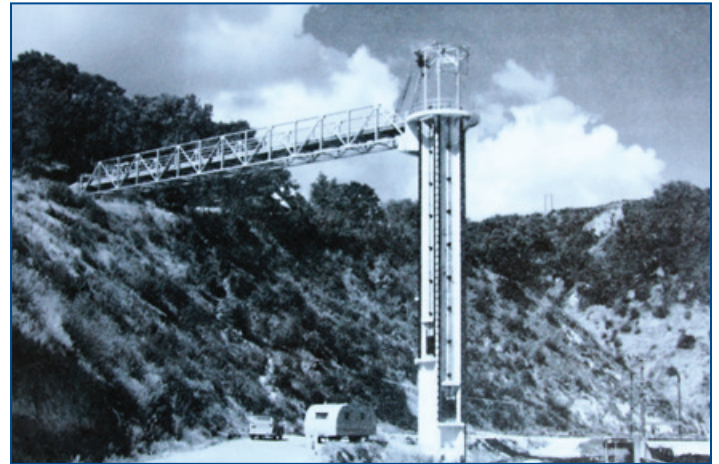
The Intake Tower at Lake Cachuma under construction in the early 1950s.
