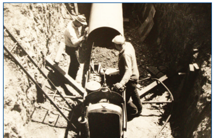
Crew members at work installing the Goleta Water District transmission main the early 1950s.
