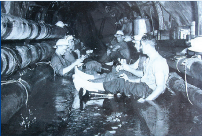
Crews building the Tecolote Tunnel take a lunch break inside the tunnel in the early 1950s.
