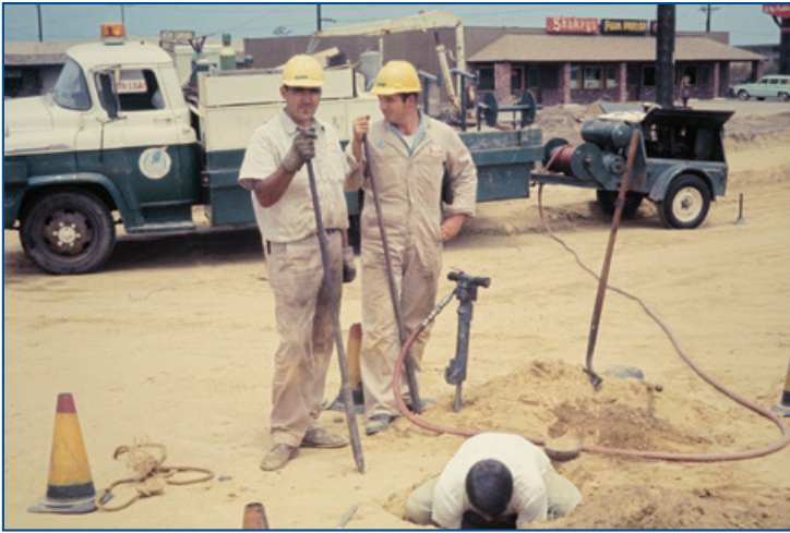
Crew members working on the Goleta Water District system in the early 1960s.
